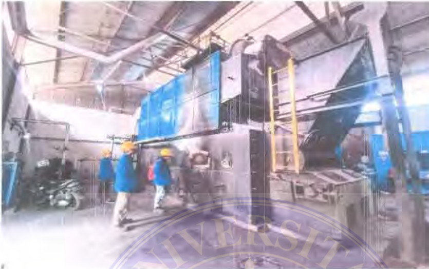
Gambar 3.3. Ketel Uap (Boiler).
