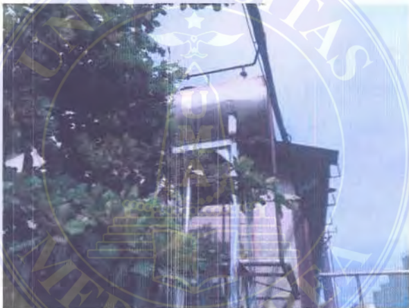
Gambar. 3.24 Feed Water Tank
