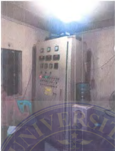
Gambar. 3.21 Panel Kontrol Boiler
