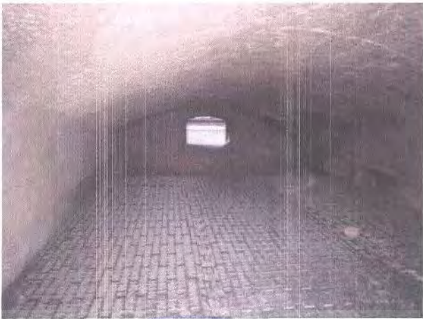
Gambar. 3.15 Ruang Bakar Boiler
