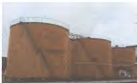
Gambar 3. 21 Storage Tank (Tangki Penyimpanan)
