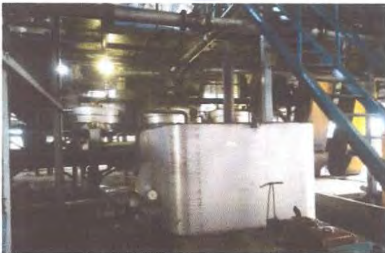
Gambar 3.19 Crude Oil Tank
