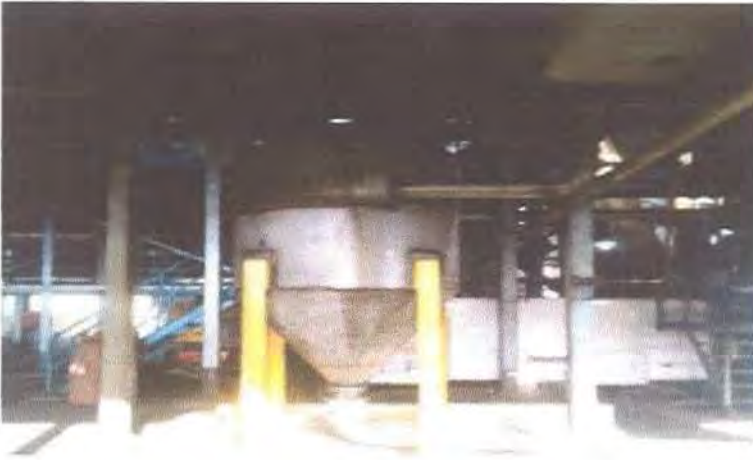
Gambar 3.4 Sand Trap Tank
