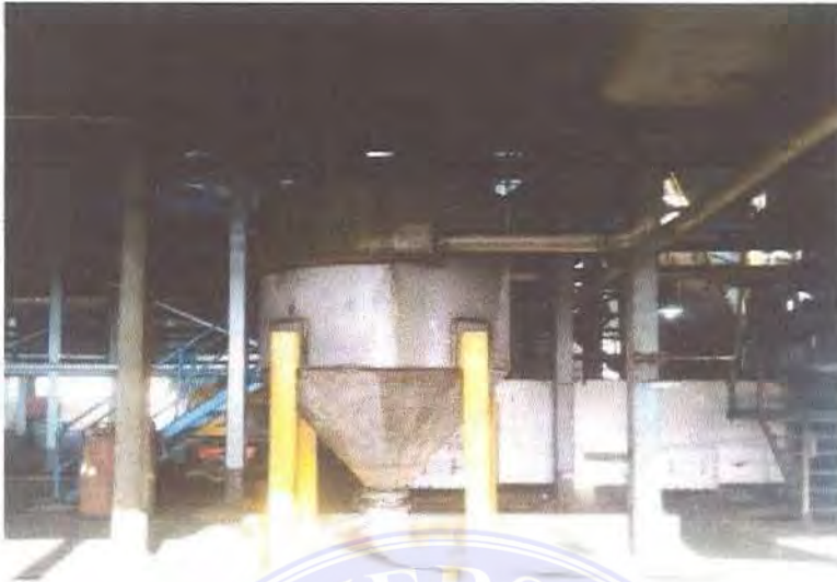
Gambar 3.18 Sand Trap Tank
