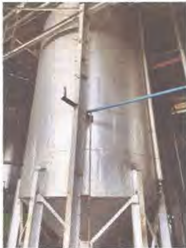
Gambar 3.12. Continuous Settling Tank
