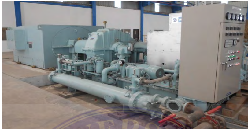
Gambar 3. 5 Turbin Generator Medan Sugar Industry
