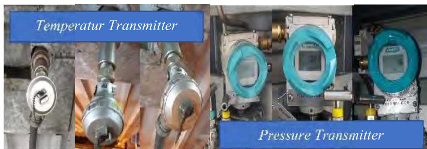
Gambar 3.4. Temperature Transmitter dan Pressure Transmitter
