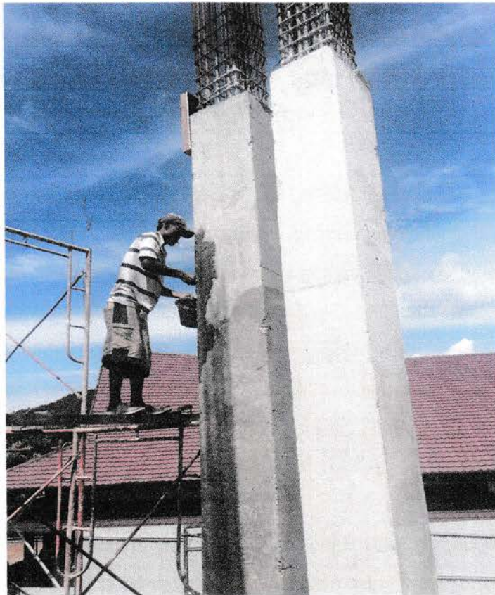
Gambar 2.4.7 Pengendalian Cacat Beton
